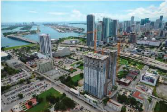
► Melo Group topped off construction at Square Station , a 710-rental unit and two 34-story towers featuring affordable rent.
